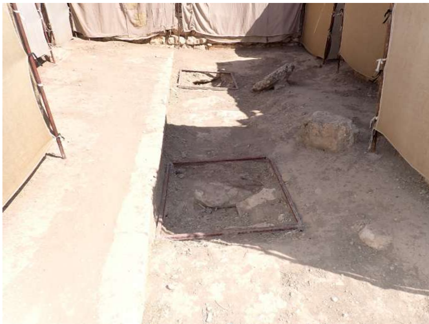
Figure 20: Image showing the missing mesh on the drainage frames in Iwan C5
